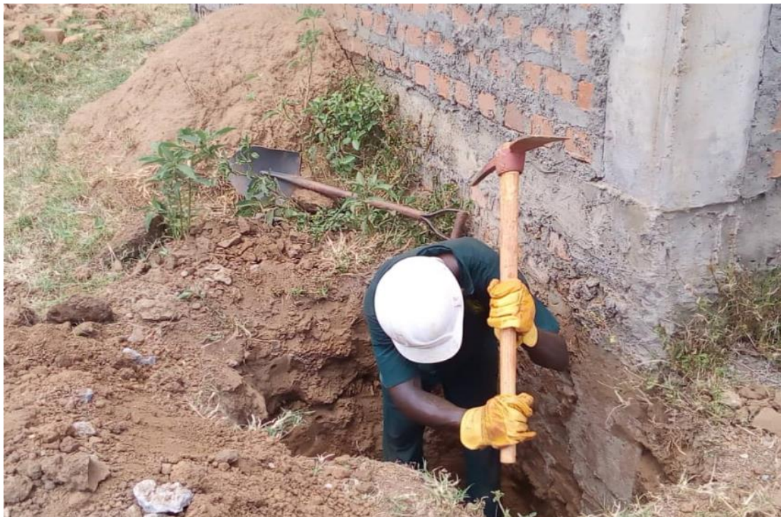
Photo plates 03: Manual excavation of test pit at one of the footing points
