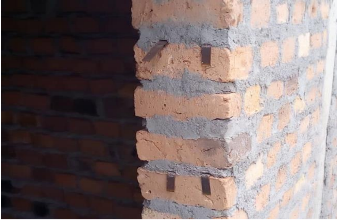
Photo plate 09: walling material used. (common burnt clay brick wall, 200mm thick)
